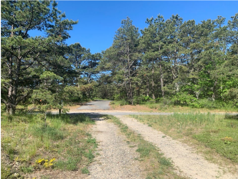
Figure 63: Road Approach (Only Paved on One Side)
