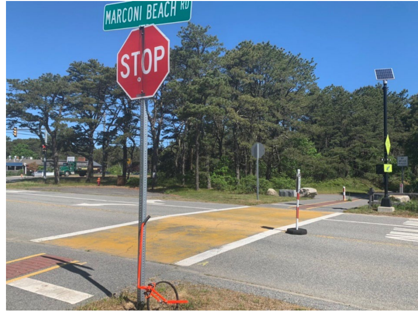
Figure 66: Faded Paint is Used on the Crosswalk. Note the RRFBs.
