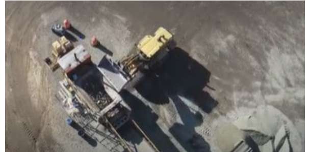
Town of Dennis Glass Crush Operation (2019)
