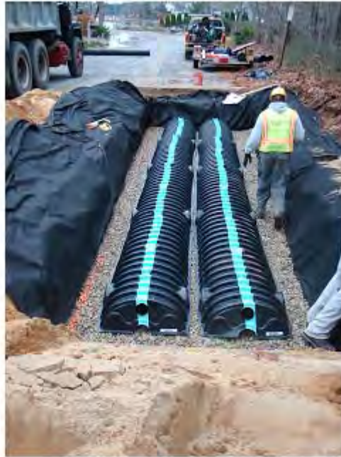
FIGURE 5: HDPE SUB-SURFACE TREATMENT CHAMBERS (PHOTO COURTESY LINDSAY COOK, CAPE COD CONSERVATION DISTRICT INTERN)
