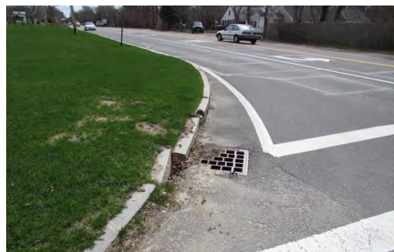
Curbing Damage on Northeastern Corner of Intersection
