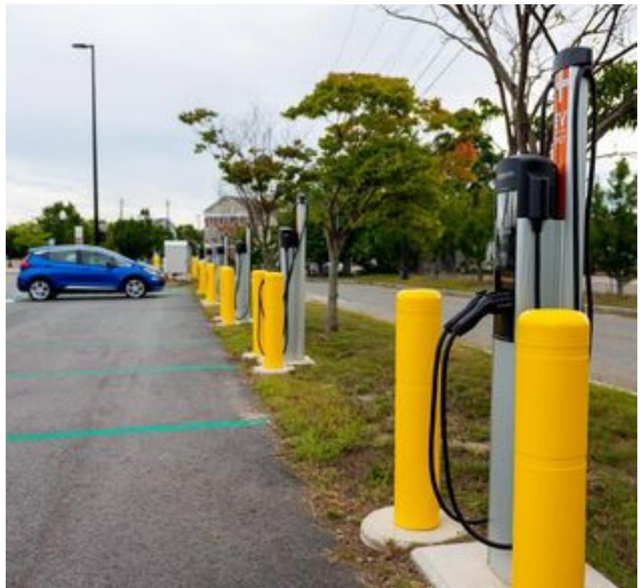
EV charging station
