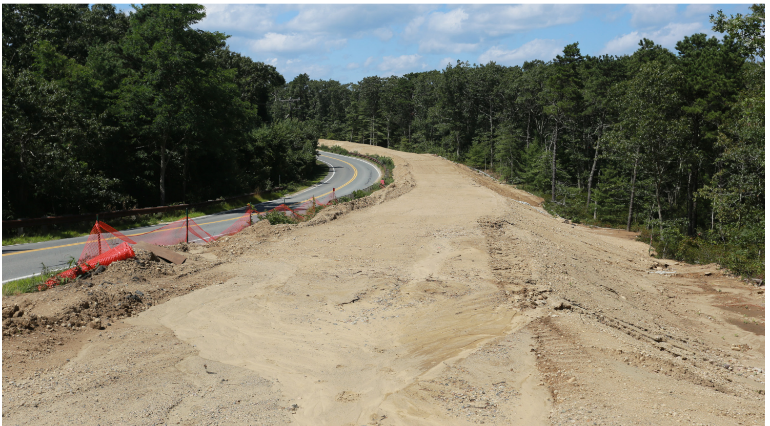
Top: Multipurpose path along Quaker Meetinghouse Road Bottom: Bike Path along Service Road under construction
