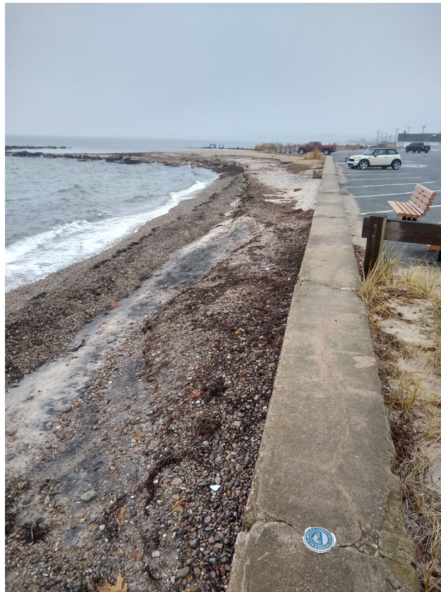
Photograph 6: Concrete seawall and coastal beach adjacent to cable landing site, facing west
