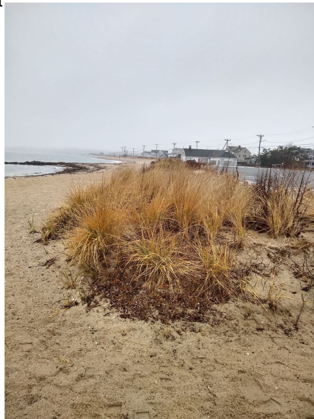
Photograph 4: Seaward edge of coastal dune adjacent to cable landing site, facing west
