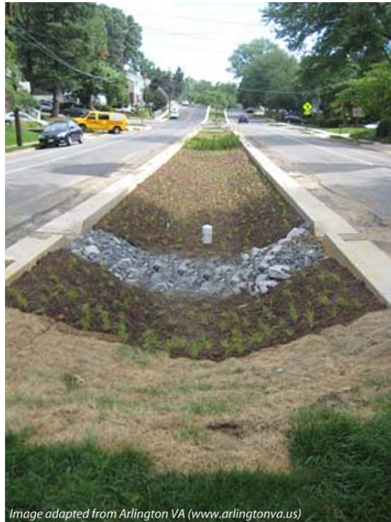
FIGURE 29 - ADAPTED IMAGE FROM THE PATRICK HENRY DRIVE "GREEN STREETS" PROJECT CONSTRUCTED IN ARLINGTON COUNTY VIRGINIA
