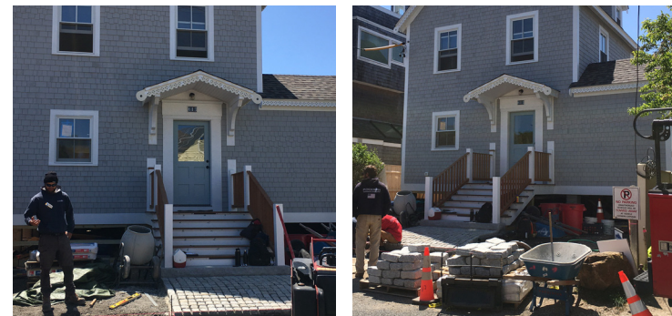
This historic structure was elevated four feet, less than would be required for a non-historic structure, in an effort to preserve the historic streetscape.
