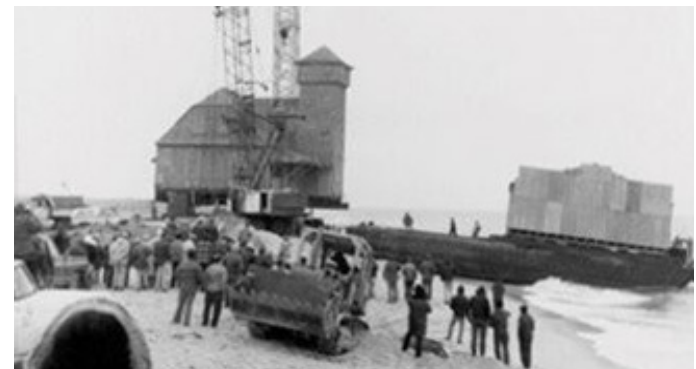
Top: Nauset Light reconstruction after being moved from Chatham in 1923. Bottom: Old Harbor Life Saving Station being moved from Chatham to Provincetown in 1977.
