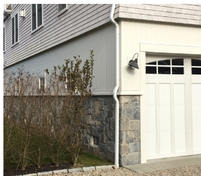
Stone facing provides a flood resistant material on wall sections that are likely to be exposed to flooding.
