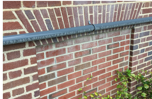
The original location and size of a basement window is preserved with inset bricks.
