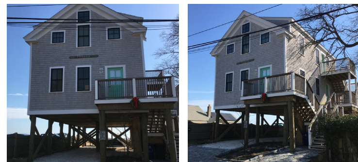
This building was originally set at the street edge but was pulled back about 10 feet to soften the impact of elevating it approximately 11 feet above its original height. The change still has a dramatic effect on the district's character.
