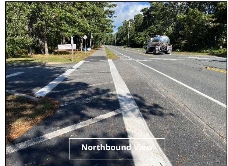
Southbound View and Faded Markings
