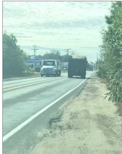
Figure 14. Current Roadway Condition
