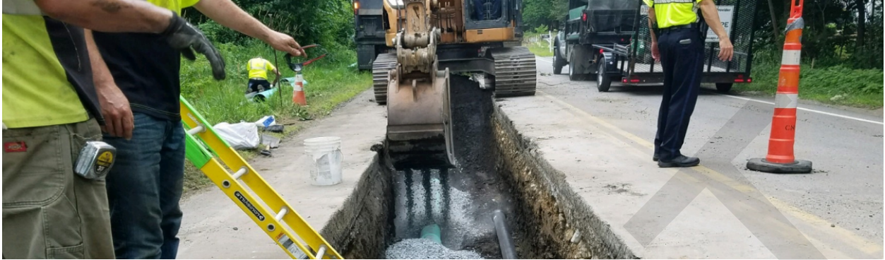
Easton, MA used DIF to install sewer lines and unlock mixed-use development.
